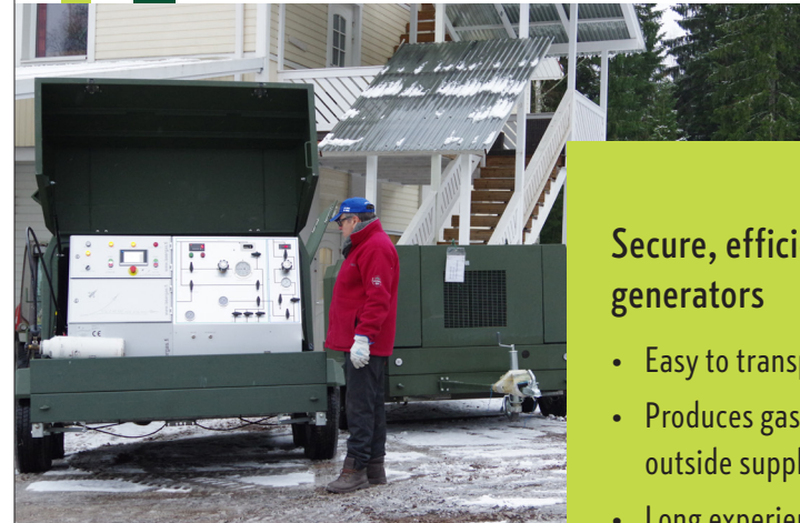
Mobil generators are easy to transport.
